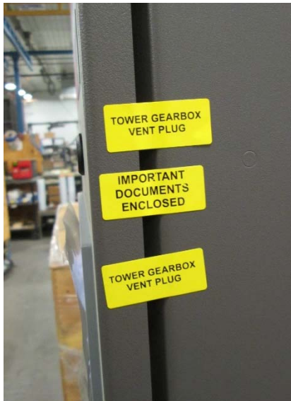
Tower Gearbox Vent Plug Located in Electrical Panel
